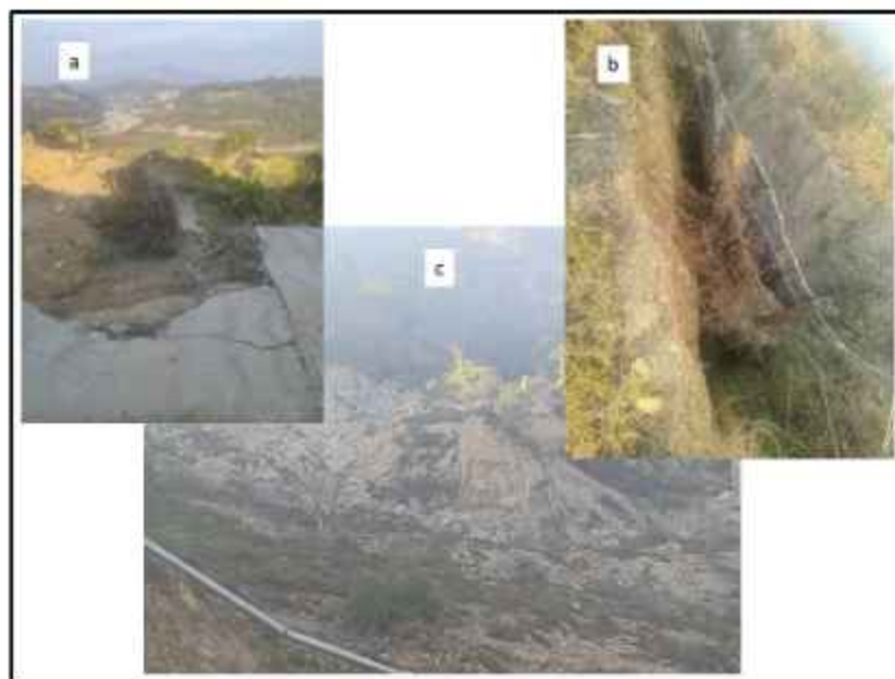
Fig. 16 a) Image depicts damage to the cemented road due to poor drainage system and b) development of wide fissure which is reminder for the next disaster. Similar features were developed on the on the displaced mass as noticed by local residents c) displaced material from the main mass and slope angle of the slide zone.
