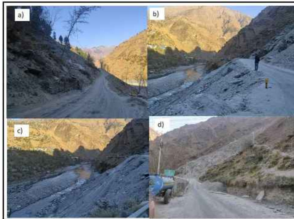
Fig.43: Lothal slide zone where presence of shear zone slope angle and water scoring action leads to toe erosion and further movement of the hill slopes and cause damage to the road.
