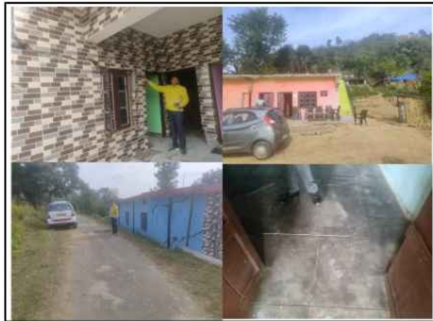
Fig. 21 Shows development of cracks in the tiles and displacement of walls b) the frontal part of the houses was totally damaged and the existing one developed wide cracks in the wall indicating subsidence cracks c) Again diagonal cracks in the walls and D) floors indicating subsidence features.
