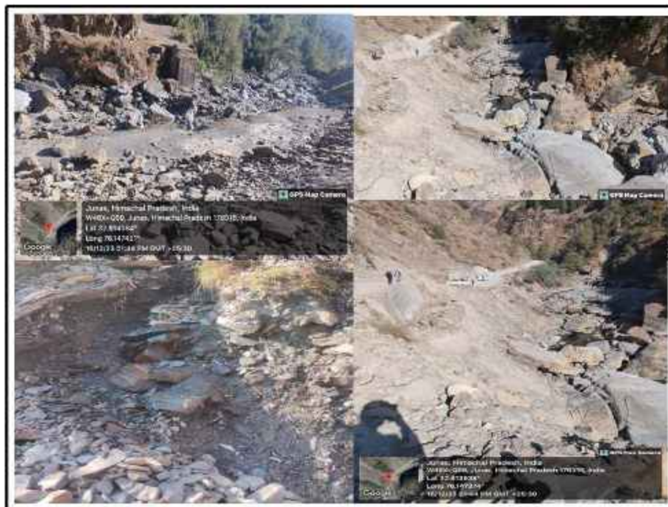
Fig.48 a) Shows the damaged part of the road and retaining wall along the Tarela-Boundary Mangli Road slide zones b & d) indicated large chunk of slates and boulders which can be used to diver the river channel and slope angle of the slide zone c) shows the moisture content and irregular stones which have been broken from the in situ rock.
