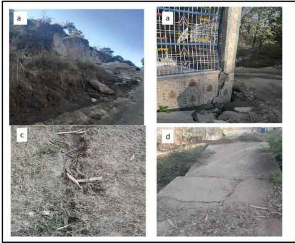
Fig. 23 Images showing hillock of the Middle Siwalik rock behind which the water was logged during heavy rain fall b) showing the damage caused to the temple due to subsurface movement. Land fissure developed in agricultural land downstream d) damage of cemented path leading to houses.
