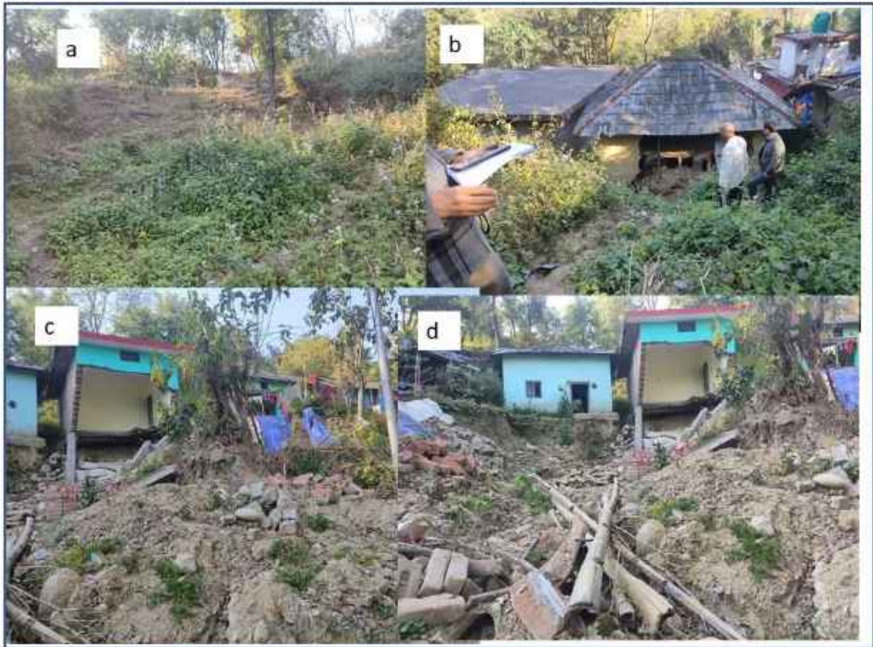
Fig. 12 Shows the damage cause to the houses in Gurthali village a) shows the slope angle and ridge from where water came after heavy rain fall b) the back side of the houses where water was blocked, the mud houses could sustain the pressure but concrete houses could not sustain the water pressure due to soft storey at the bottom c and d) damage cause especially removal of lower portion of concrete house and havoc caused by blocked water in the down side agricultural land in front of the houses.
