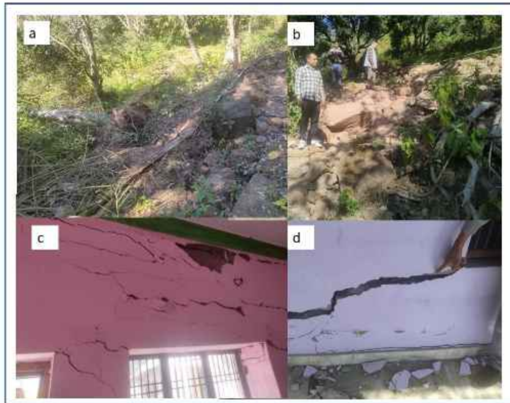
Fig.14 Uprooting of trees and displacements of roads and it's downwards movement suggesting deeper slip surface b) Development of cracks in walls suggesting movement direction
