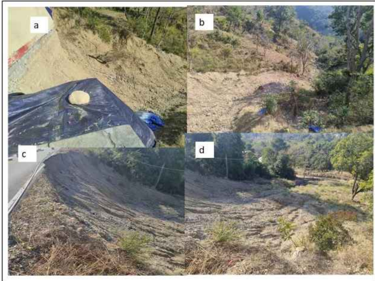
Fig. 11 Shows the lithology of the slide zone, characterized by gravelly soil, is evident in the displacement of the retaining wall observed on the upper right-hand side, which occurred due to the combination of heavy load and rainfall on August 14, 2023. The upper left photo illustrates the slope angle and pattern, while the lower picture depicts a slide along the National Highway in the same village, just a few meters downstream. Once more, the inability of the lithology to withstand the high moisture content in the gravelly soil resulted in a loss of frictional strength, leading to downslope.
