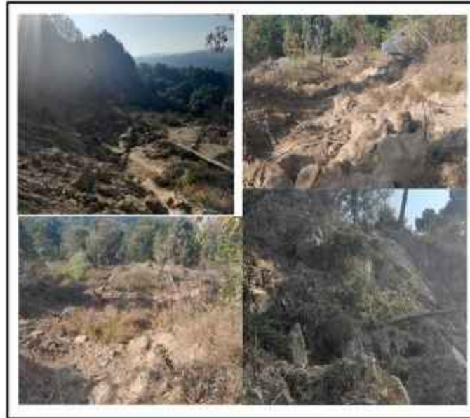
Fig.25. Shows the damage in lower Mard village hillock due to high intensity rainfall, uneven topography, uprooting of tree and developed of crevasses and depression indicated the pressure of rain fall on 14 th August 2023.
