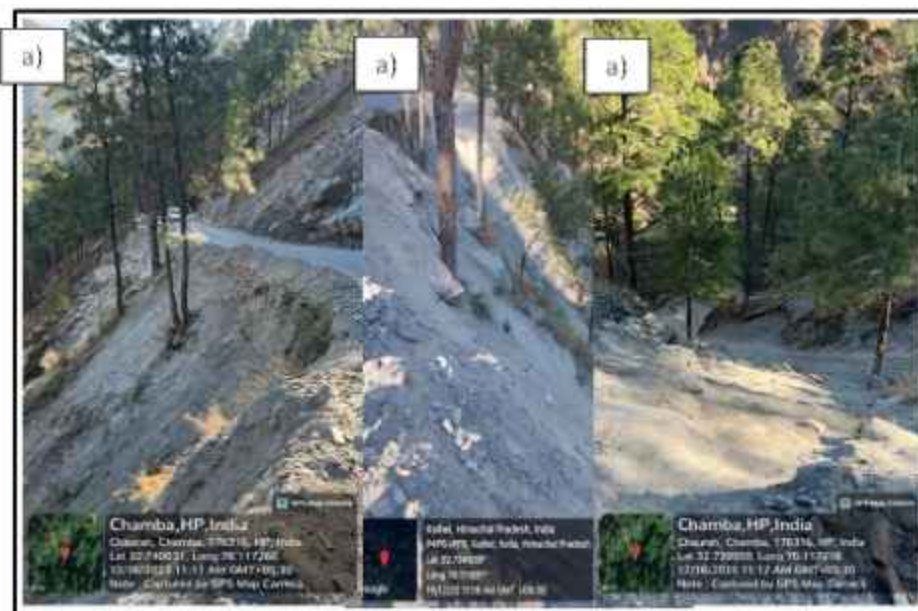
Fig.46: Image depicts a) leeward side of the road where hard rock dipping towards hillock can be seen which can be used to raise the protection and road widening wall b) slope angle and the pulverized material located at MDR 85 site c) the slope angle at the lower part of the slide zone
