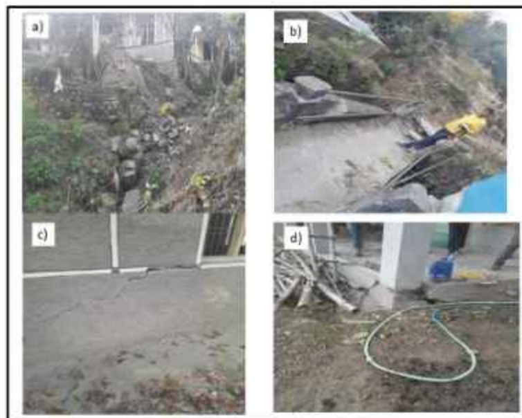
Fig. 29: Shows damage cause in the middle part of the slide zone to housing and erosion of the retaining walls along the natural drainage b) damage of cemented path c) development of cracks in building d) displacement of pillar and damage caused.
