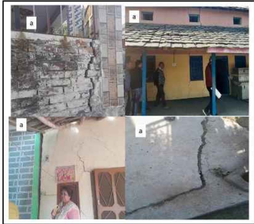
Fig.26. Shows subsidence crack in walls, and roads due to water logging and poor drainage system in the village. No doubt high intensity rainfall contributed to the damage but the moisture already present in the soil got accelerated by high intensity rainfall and thus developed subsidence crack at Pokhru village.
