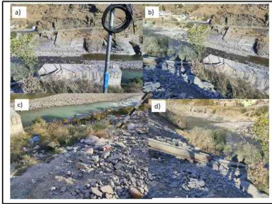
Fig. 42 Image depicts a) damaged retaining wall raised within the water body due to subsidence of the foot of the wall b) Damage to the retaining wall on right bank of the river c and d) area river and road indicating enough space for raising protections walls.
