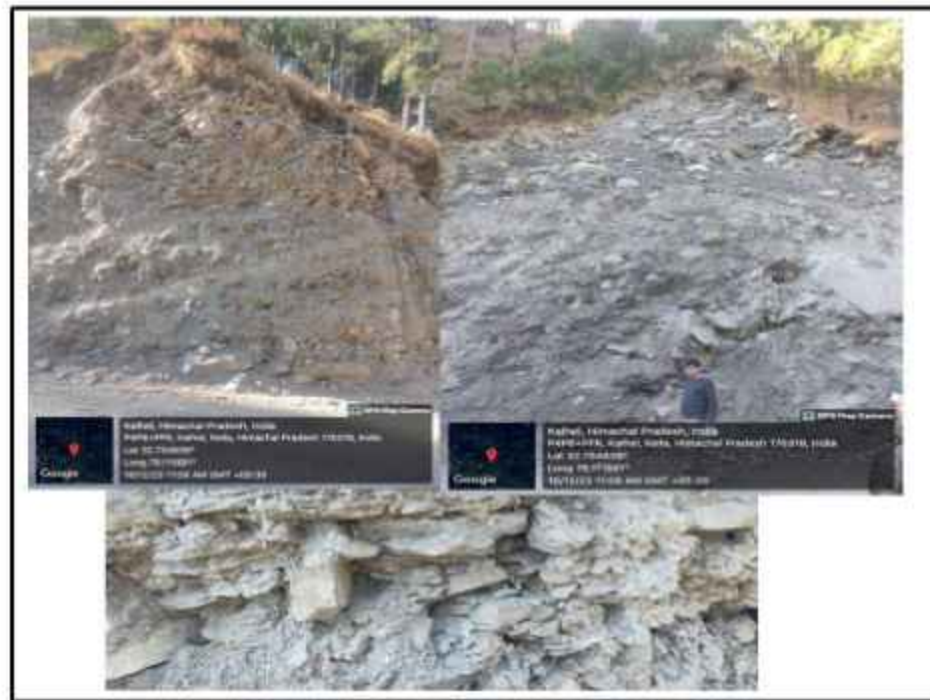
Fig.45 Image depicts a) highly shattered phyllites rocks with number of joint planes which are subjected to high stress due to presence of tectonic plane in its vicinity b) shows the upper reaches of the MDR 85 sites with very loose material which can move downslopes under high moisture condition due to its low frictional strength c) Phyllites rocks with number of joints and sheared adjacent to the MDR 85 site.
